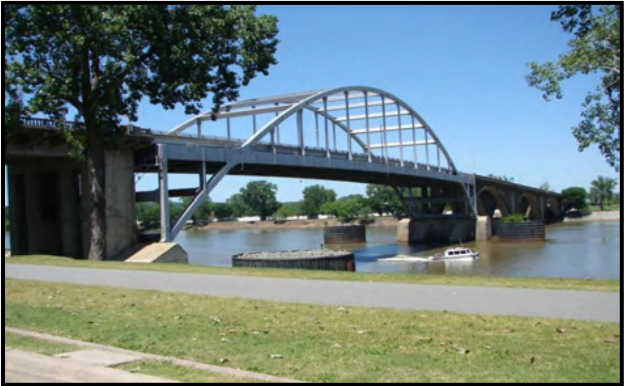
Figure 21. View of the Broadway Bridge from the Arkansas River Trail, LR side
